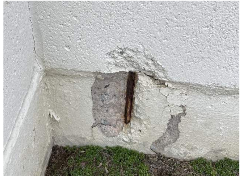
Exhibit #2: Exposed reinforcing
