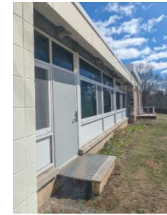
Landing and step at classroom door riser height exceeds code requirements
