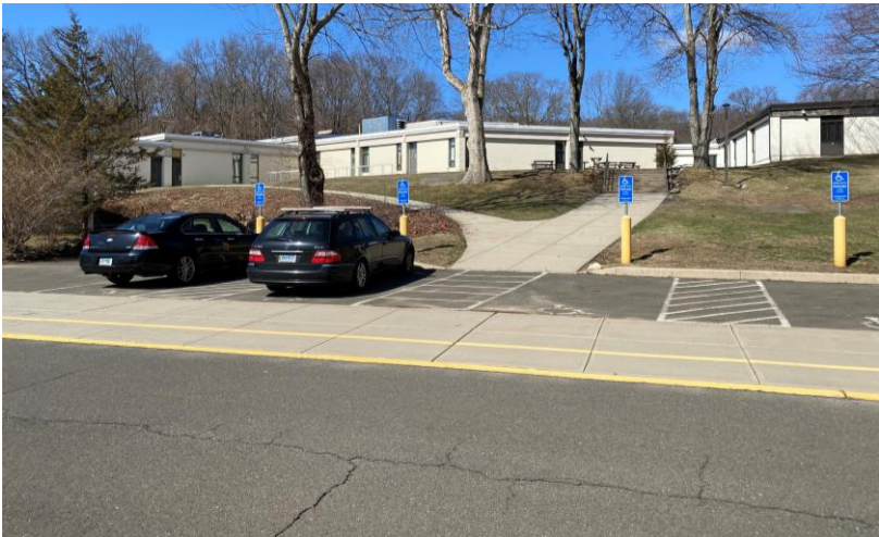
Accessible parking at the south parking lot. Visible alligator cracking.
