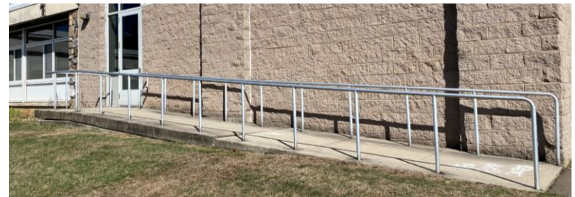
Non-compliant ramp at the Library
