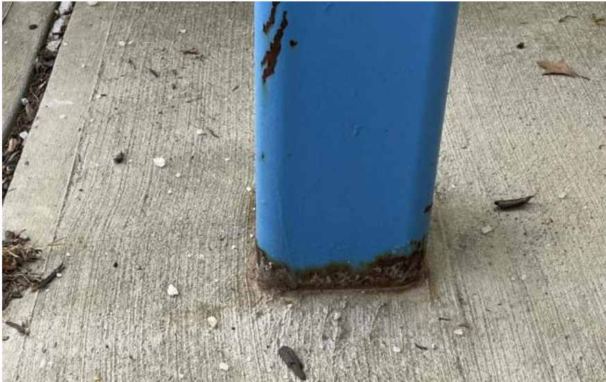
Exhibit #23: Surface corrosion at base of canopy column
