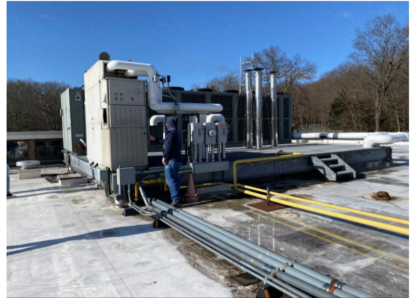
Rooftop chiller and microturbine
