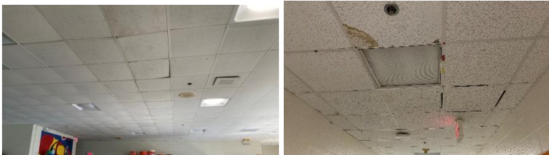
Dirty and sagging ceiling tiles
