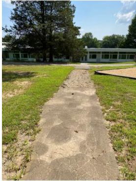
Sidewalk in need of repair
