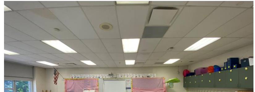
Typical 2x4 ACT ceiling in a Classroom
