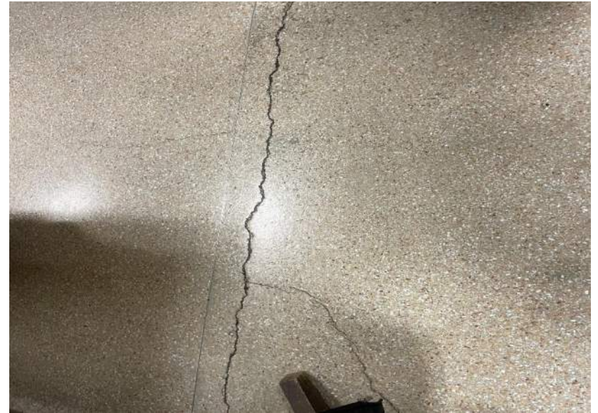
Exhibit #11: Cracking and heaving at slab on grade
