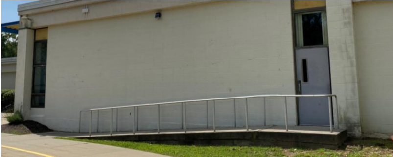
Non-compliant ramp at the South Assembly
