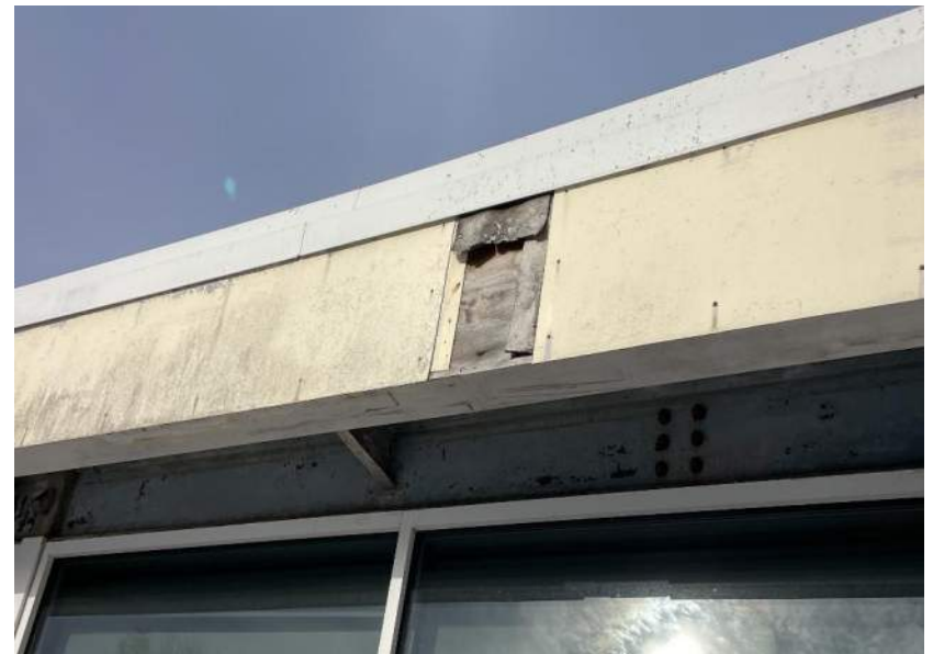
Exhibit #22: Exposed steel at soffit
