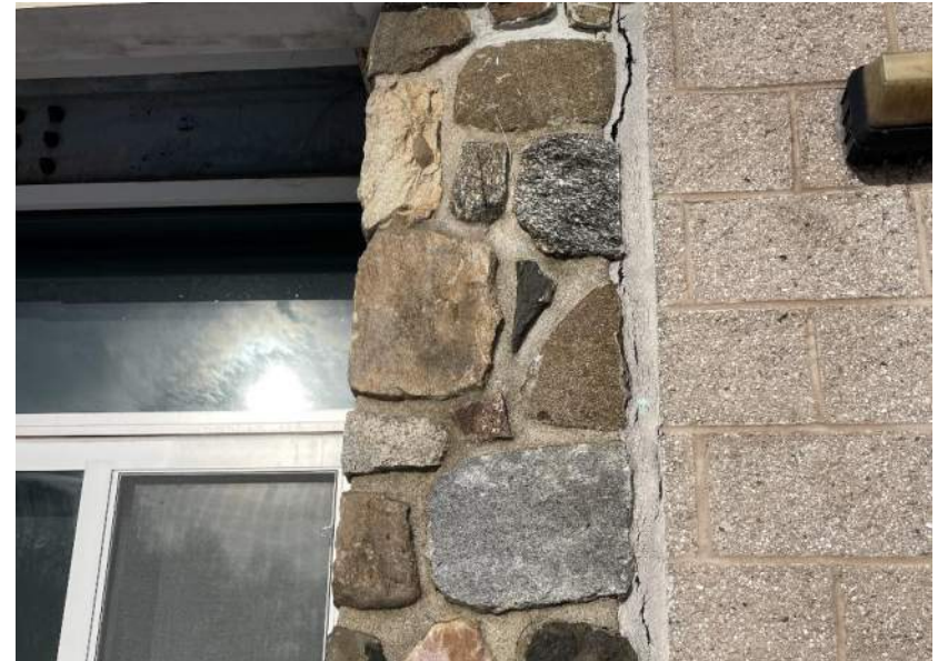
Exhibit #26: Joint sealant failure (typical)
