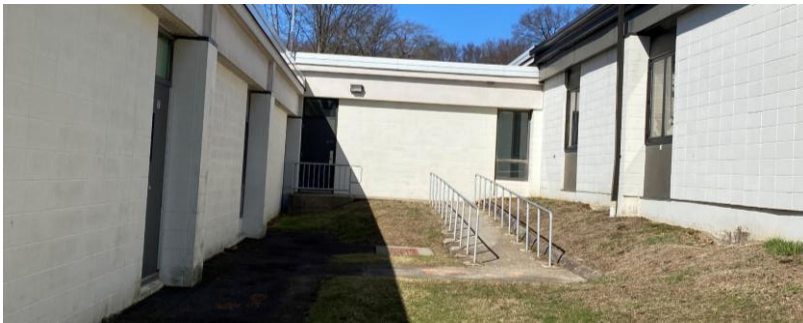
Non-compliant ramp between the 1970 and 1994 addition
