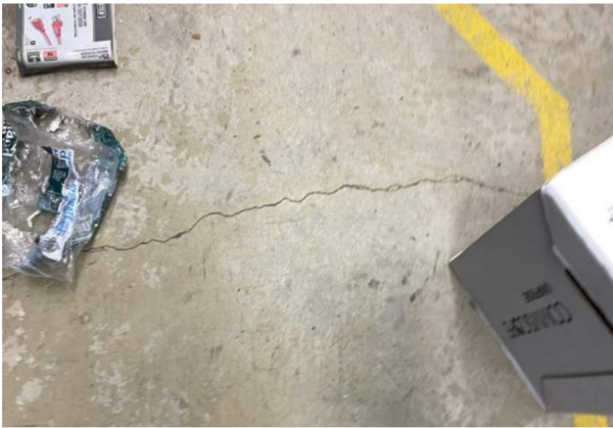
Exhibit #14: Slab on deck cracking at mechanical room
