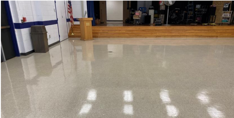
VCT flooring in the South Assembly Room. Typical to Classrooms, as well.
