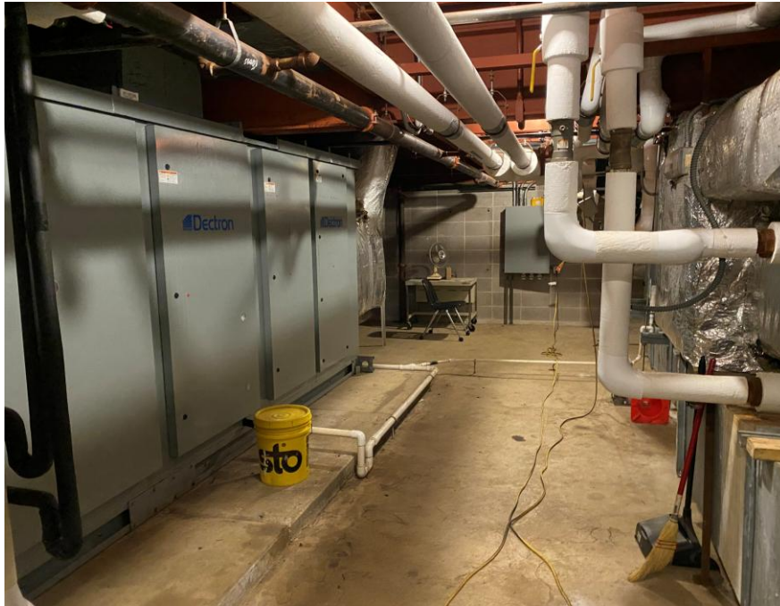
Unit and ductwork serving pool area.
