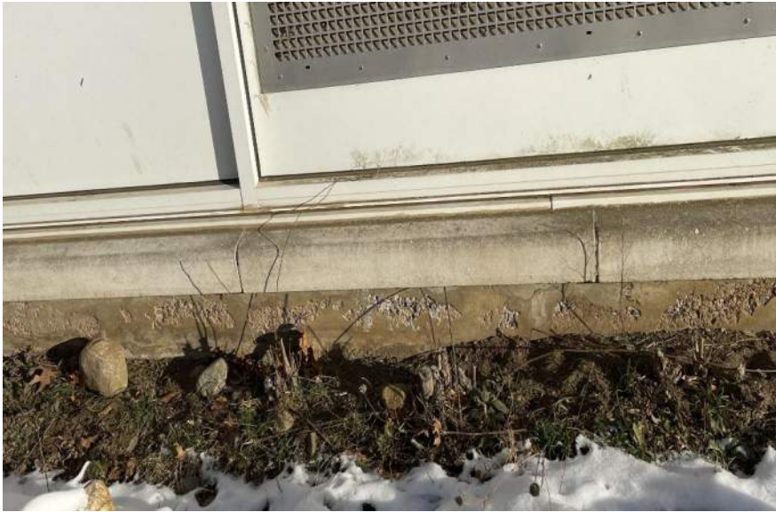
Exhibit #7: Exposed aggregate and deterioration
