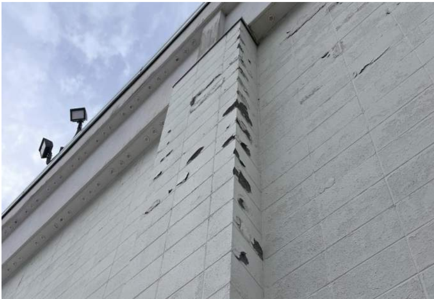
Exhibit #20: Spalling and separation of CMU at pool
