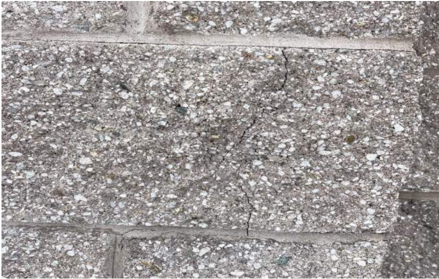
Exhibit #19: Cracking at split face CMU (typical)
