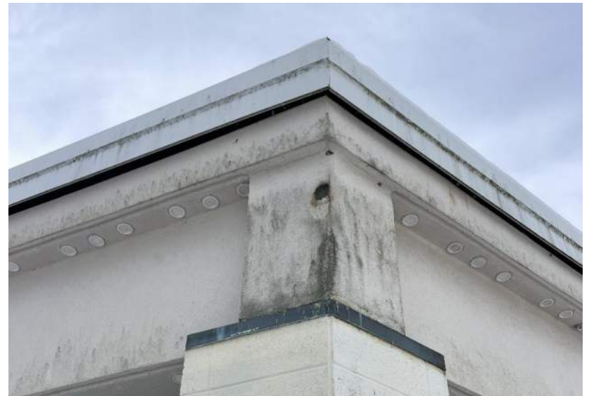
Exhibit #29: Damaged EIFS (typical )
