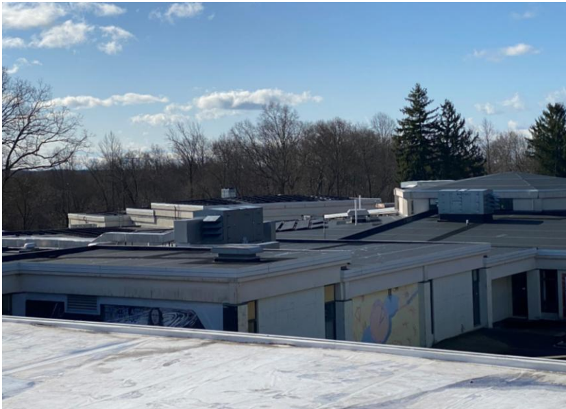
View from North wing rooftop showing multiple rooftop units, ductwork runs above roof deck, and solar panels beyond.
