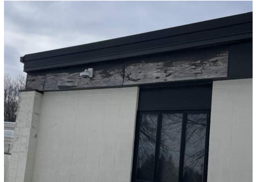
Exhibit #28: Exposed sheathing at soffit
