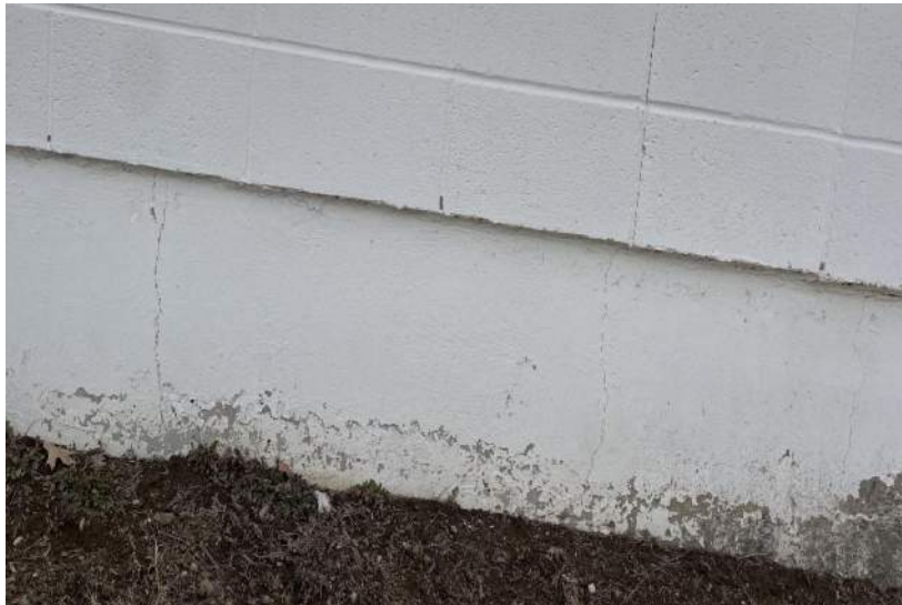
Exhibit #1: Foundation Cracks Typical
