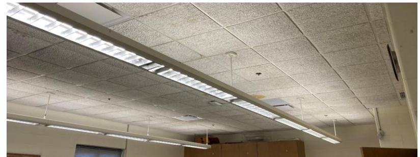
Typical 2x2 ACT ceiling in a Classroom
