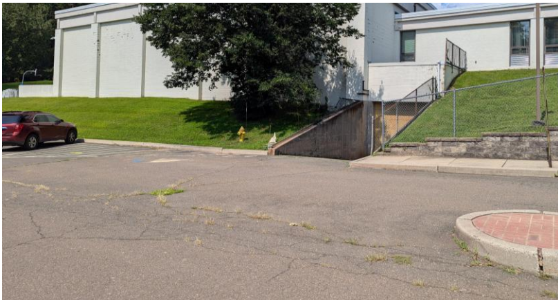
Visible alligator cracking and organic growth. South parking lot.
