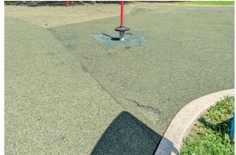
Cracking and wear at rubber playground surface
