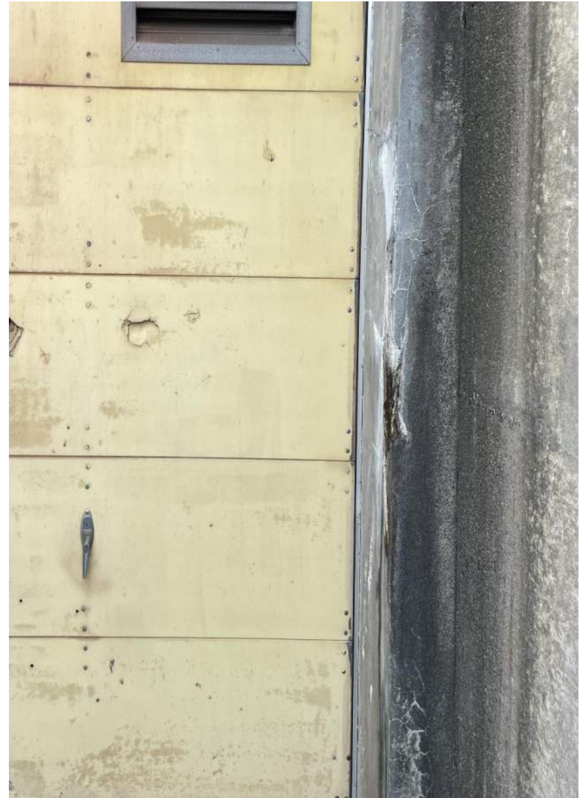
Exhibit #9: Severe cracking and delamination
