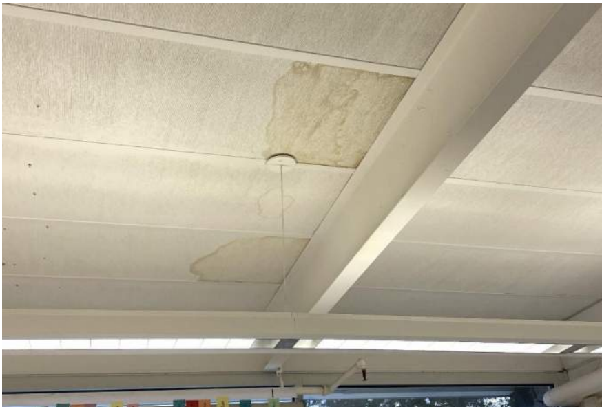
Exhibit #24: Interior water damage (typical)
