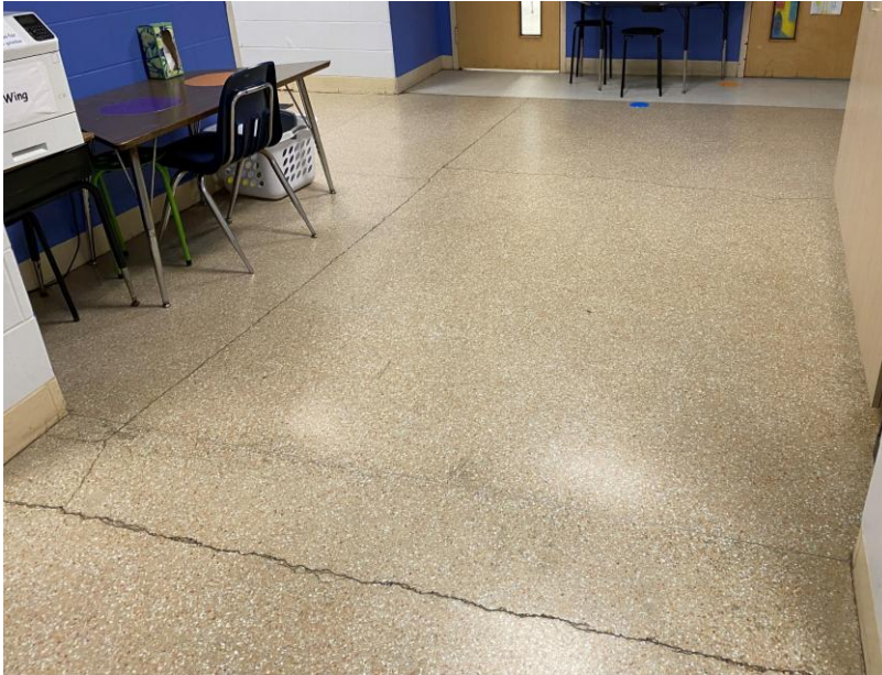
Cracked terrazzo flooring, 1960/64 portion of the school
