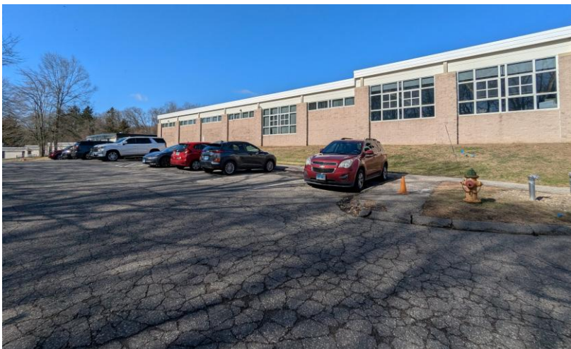
Visible alligator cracking in the paving. Mid-level parking lot.
