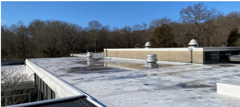
Ponding water on the 1960/64 wing
