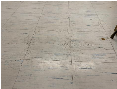
Cracked VCT in the 1994 addition
